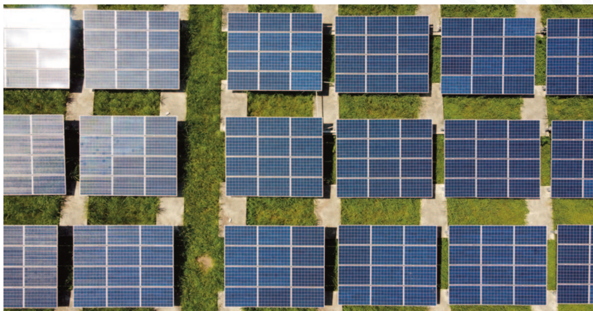
2 MW, Taipei Energy Hill, Taiwan.
