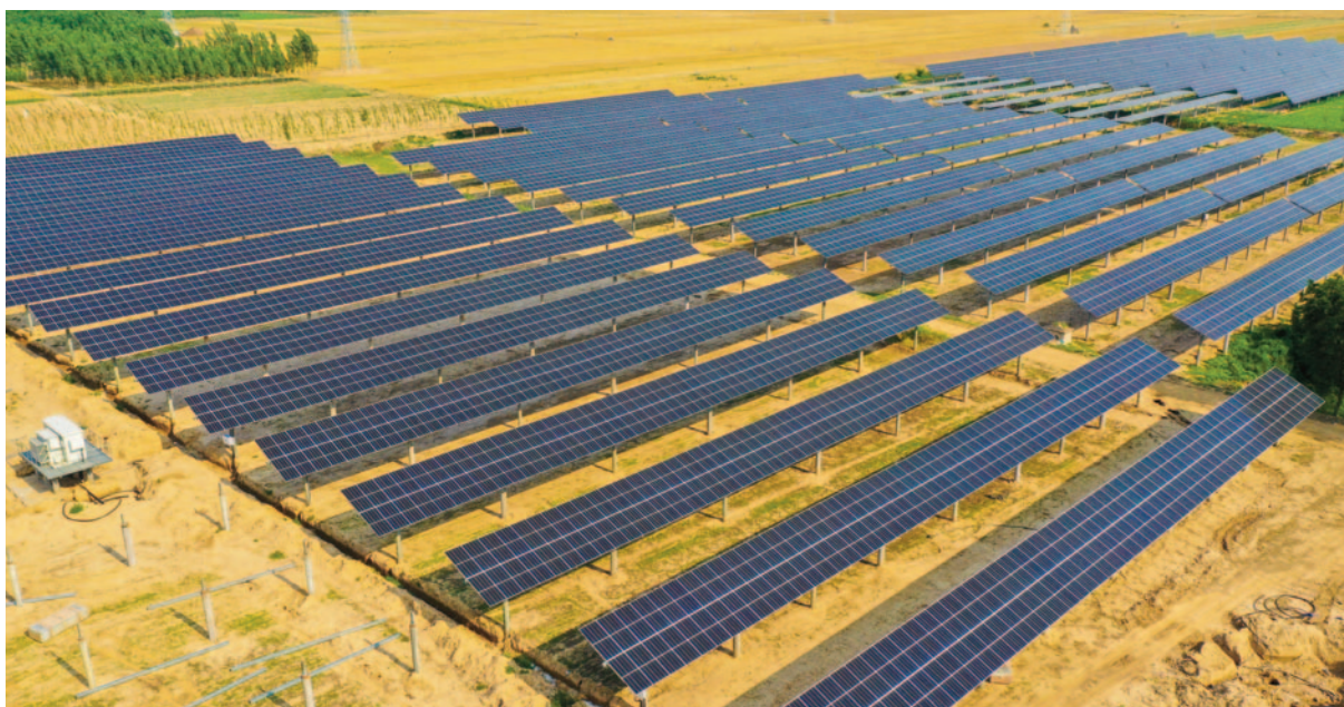
400 MW, Nangong, HeBei Province, China.
