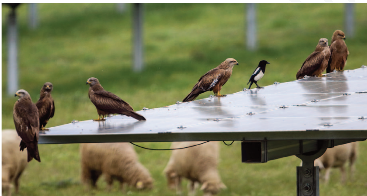
50 MW, Solanilla, Trujillo, Spain.
