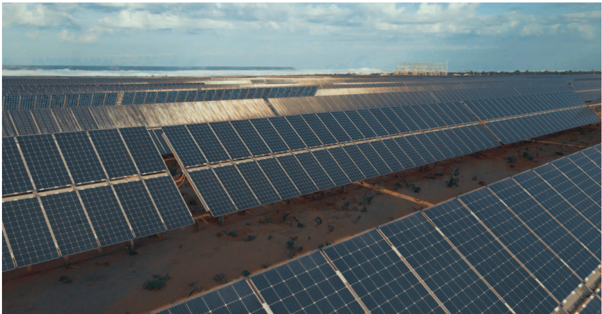
São Gonçalo solar park, Brazil.
